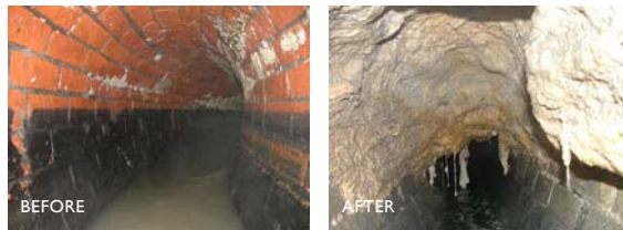
The effects on the sewer network of FOG:
